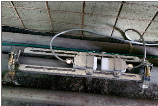
Food industry – pure water boiler pipe
